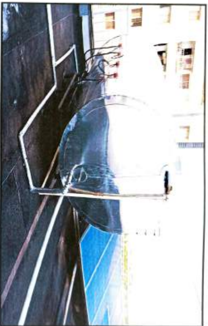
Hot Water Solar System at Hostel
