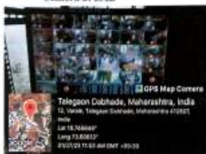
CCTV Access at Server Room
