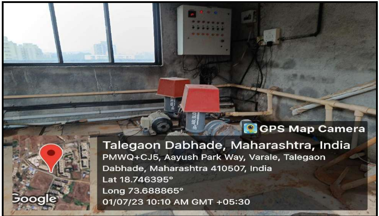
Motors, other Equipments in Disposal System and Tank
