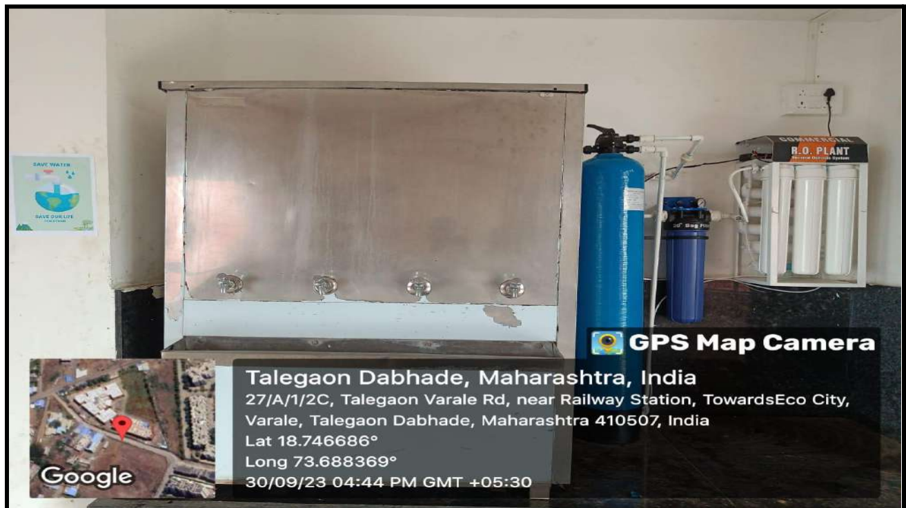
RO water plant
