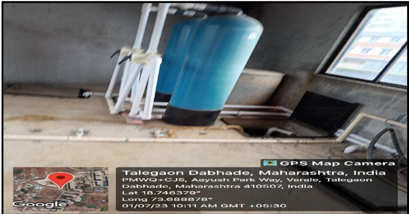
Water Treatment System
