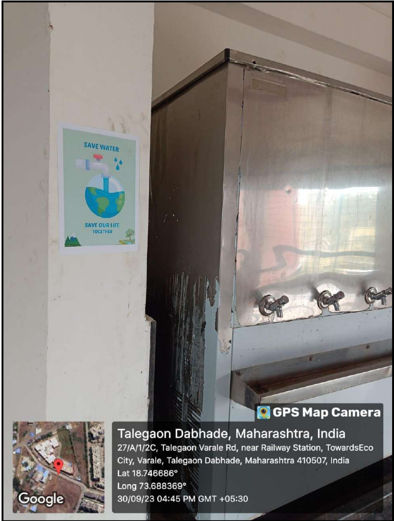
RO Water at Institute
