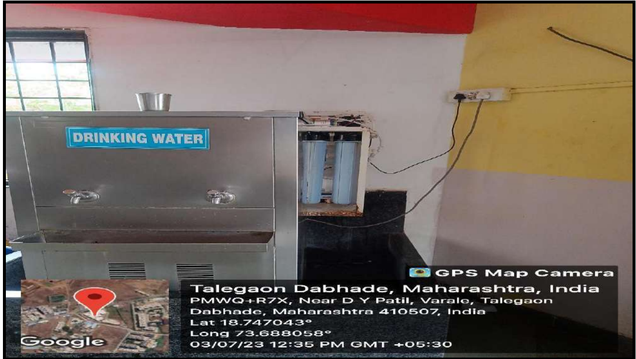
RO Drinking Water Facility at Canteen
