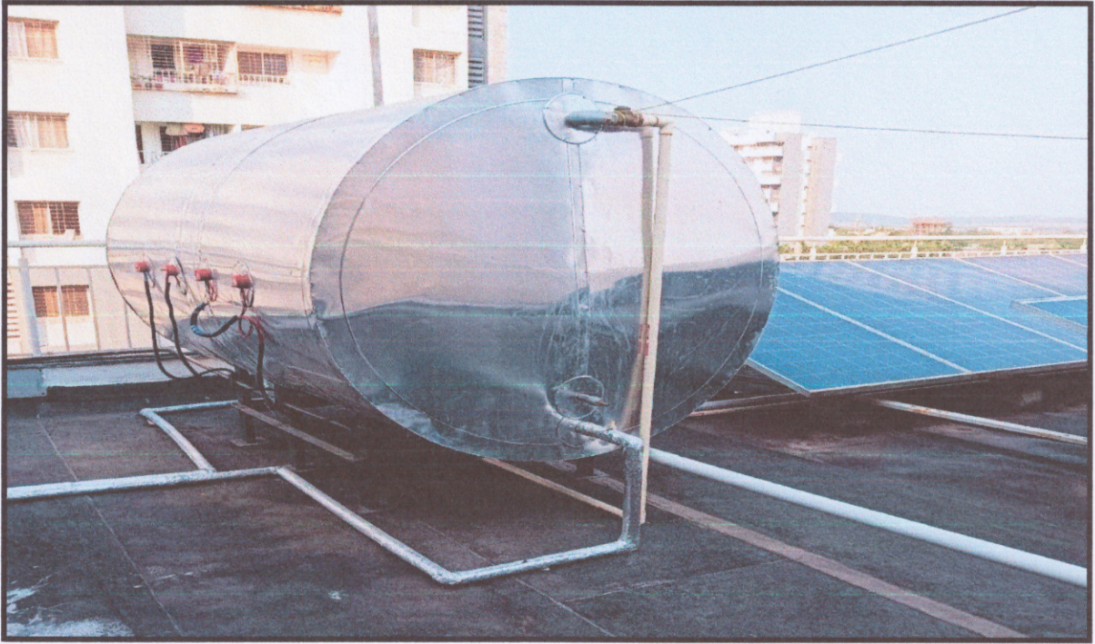
Hot Water Solar System at Hostel
