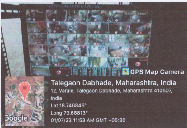
CCTV Access at Server Room
