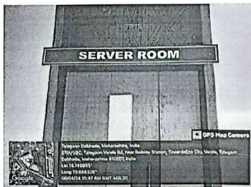
Server Room for ICT Management
